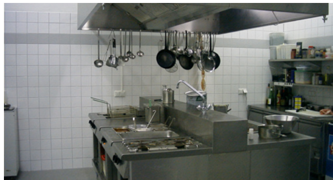
Filter monitoring in kitchens
