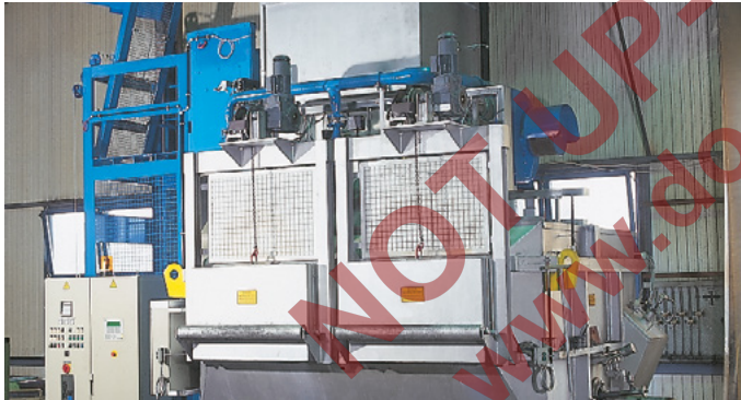
Aluminium industry: shaft melting furnace
